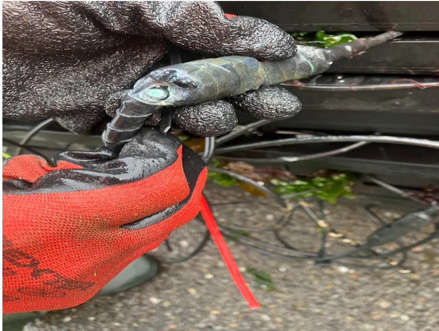
Figure 11. Corrosion damage to a standard MC4 connector exposed to saline marine conditions, showing copper oxidation (“green rot”) and insulation degradation caused by salt aerosol ingress, thermal cycling, and DC-induced electrochemical reactions.
